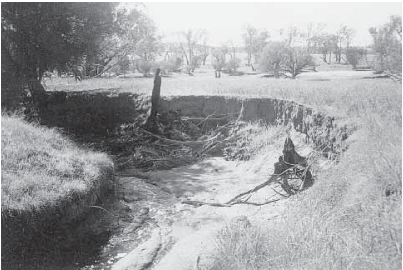
Photo 9: Active erosion of the Breckna Brook channel on the river floodplain
