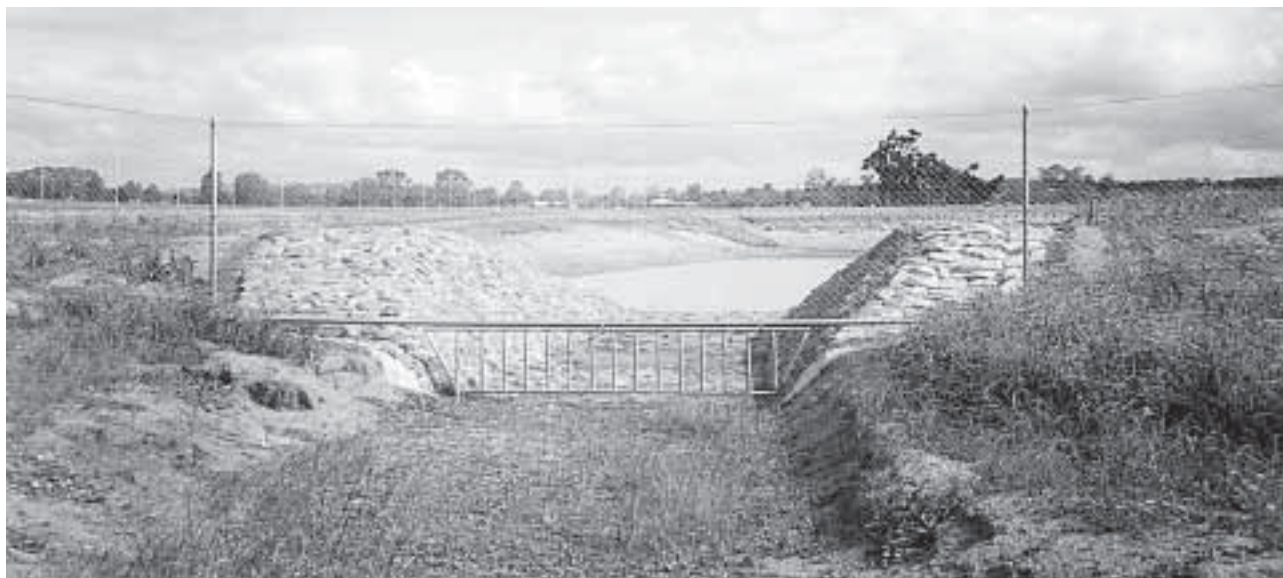
Photo 19: Detention pondage for rural-residential development near York
