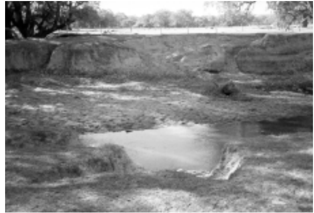
Dandalup River, Pinjarra - typical river bank degradation, bank erosion and slumping due to lack of vegetation and cattle trampling.
