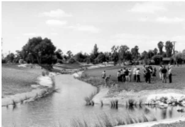
Figure 3. An example of a living stream - Bannister Creek, Perth - An urban stormwater drain (L) was streamlined using river restoration techniques (R). Large volumes of soil were removed from the site to 'meander' the creek and reshape the steep banks to a gentler slope, suitable for planting. Riffles were built to aerate flows and create habitat. Erosion control matting was used to stabilise sections of the stream banks and the area was revegetated.
