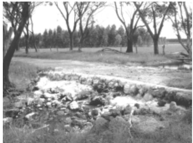
Figure 6. A causeway showing ongoing attempts to stabilise the erosion caused by floods overtopping the road and water jetting through culverts.
