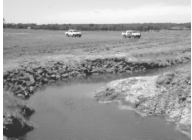
Figure 22. Bank armouring. Note that armouring a bend with rock, for low flows, may aggravate turbulence and erosion during high flows.
