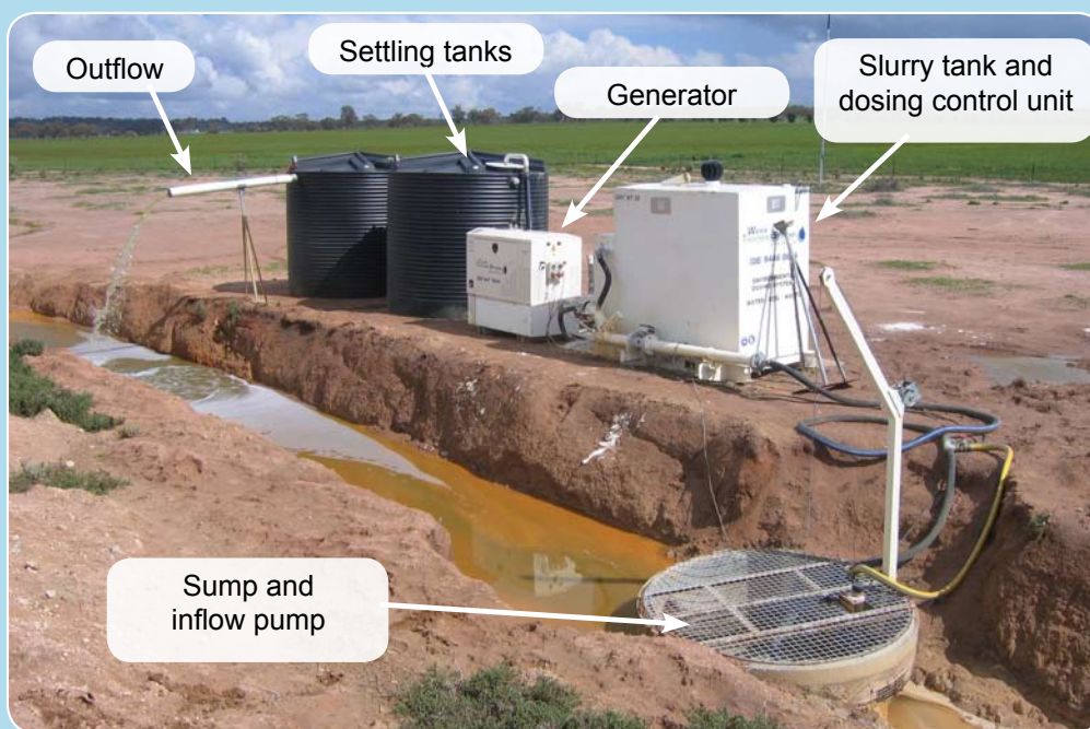
Figure 1 Hydrated lime dosing plant treating water at the end of the deep drains in the Wallatin Creek catchment
