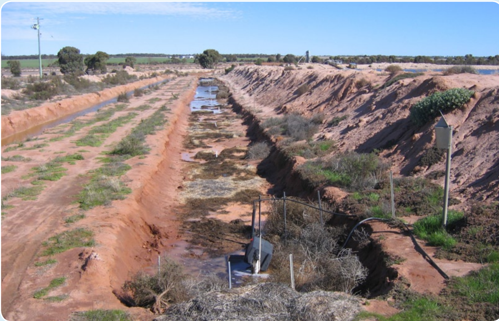
Figure 3 A composting bed in a pit constructed at the end of a drain near Beacon
