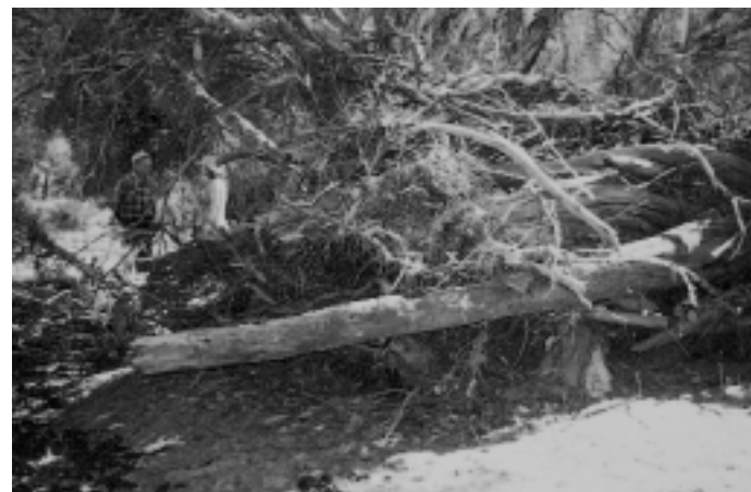
Debris from upstream creates a problem for downstream landholders when it diverts flow away from the main channel.
