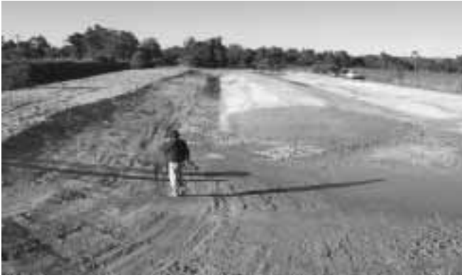
Figure 22b. Treatment channel built adjacent to the main Punrack Drain, site B.
