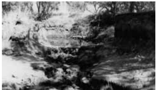
Figure 1. Spencers Brook prior to restoration works. The base of the brook is severely eroded and the headcut is actively advancing upstream.
