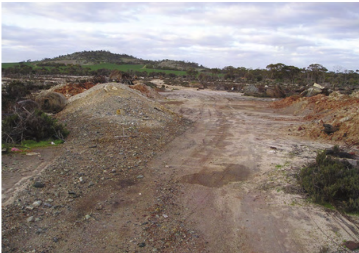
Photo 7 Road construction and rubbish at the upstream end of the site
