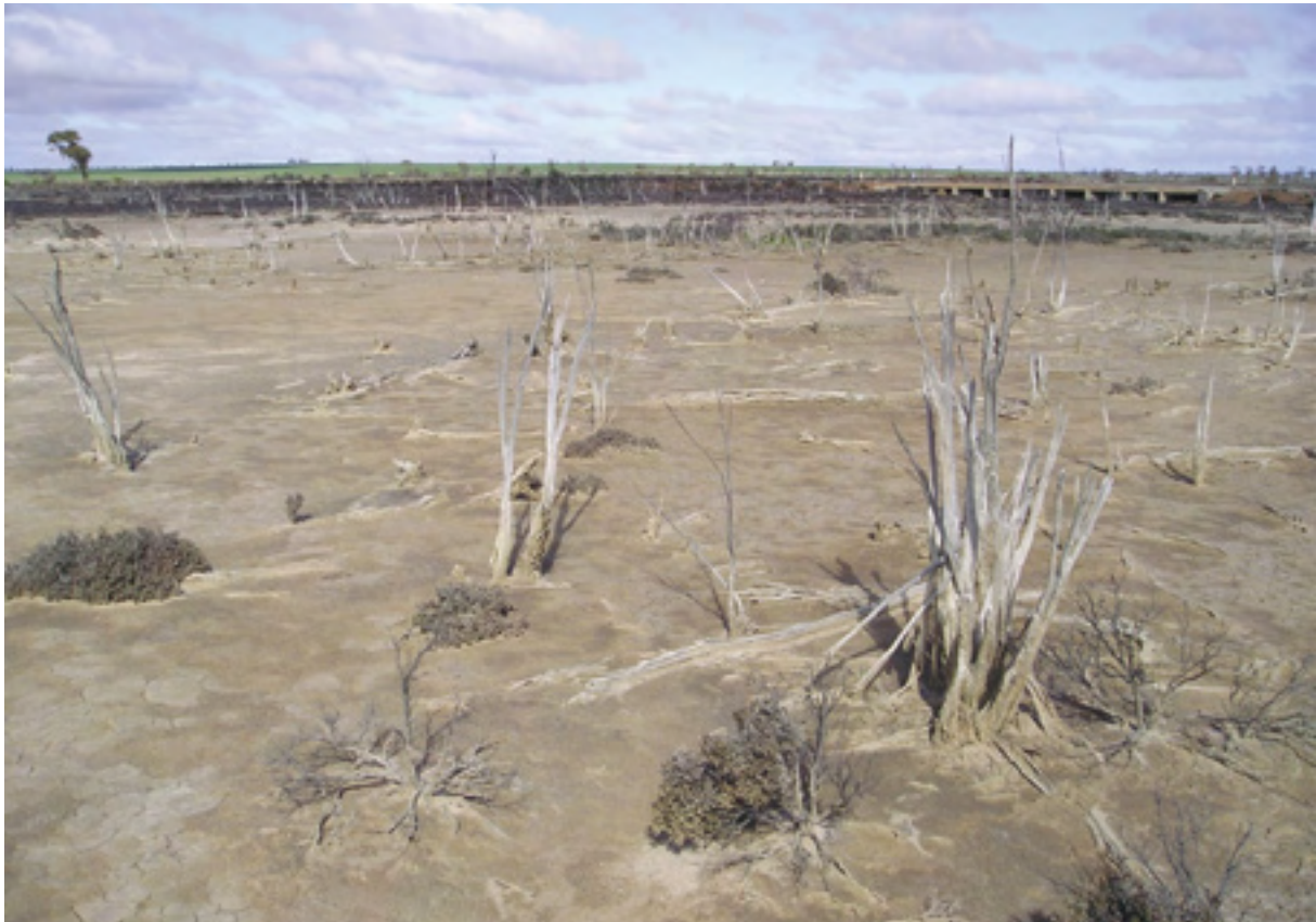
Photo 32 Broad eroded main flow channel with Bruce Rock-Corrigin Road culverts
