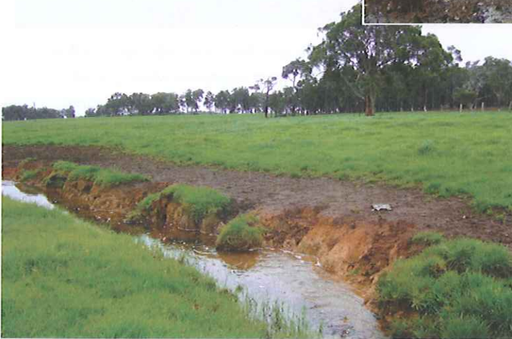
D2 grade foreshore: Stock have created a track on one side of the channel. The channel is freely eroding.
