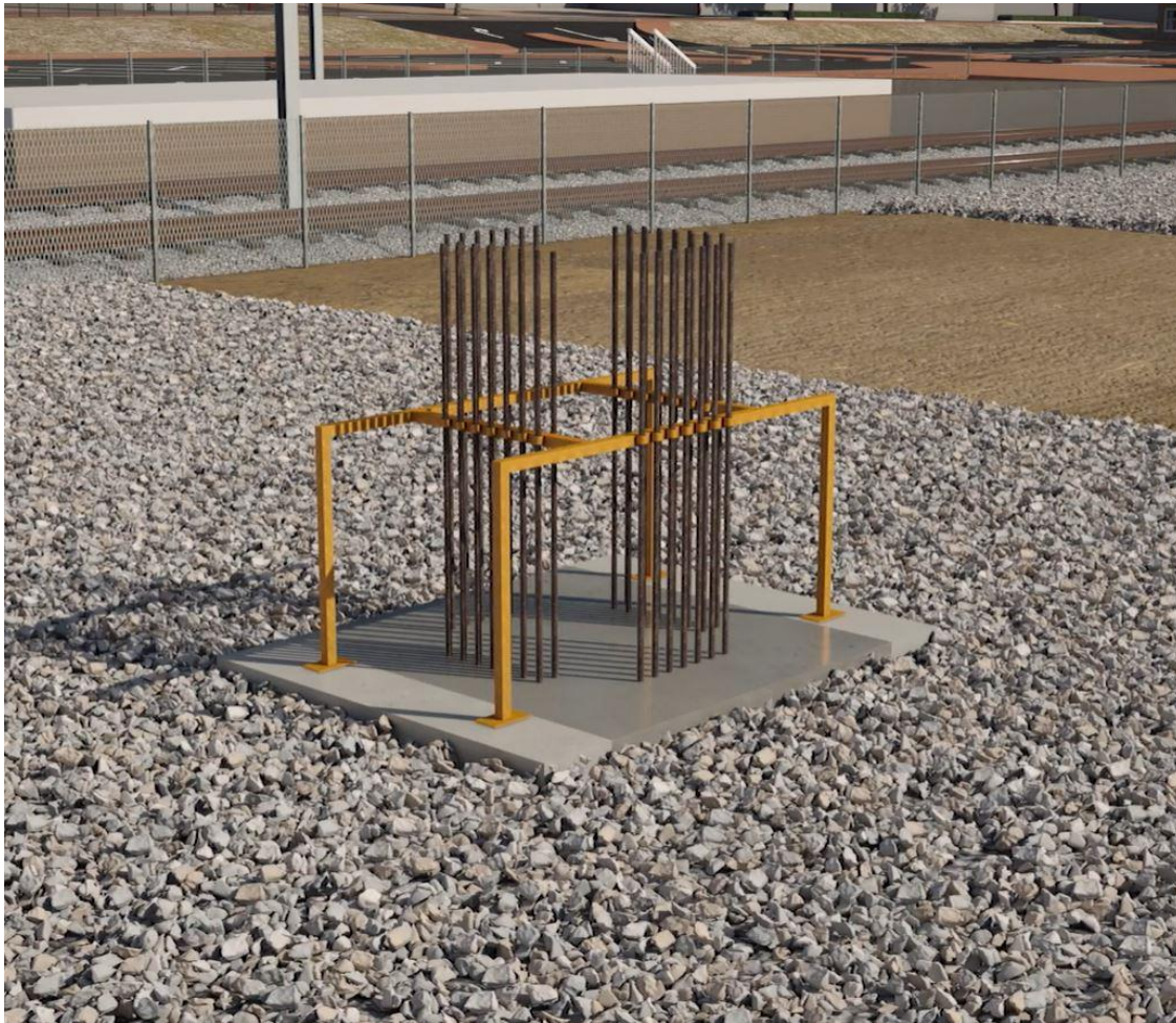
Figure 14: Example of Viaduct Column Starter Bars Set into Top of Pile Concrete Using a Steel Jig
