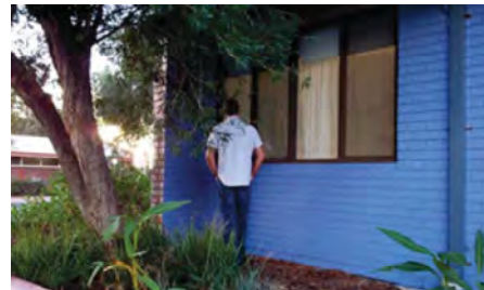
Flora conceals potential legitimate behaviour and lighting. Potential climbing aid. Poor lighting.
