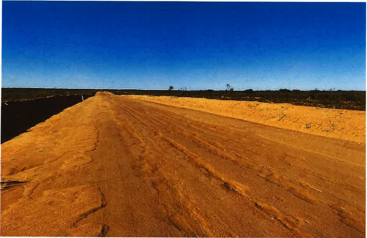
Minor erosion in sandy section of road at about 29km mark after heavy rainfall event
