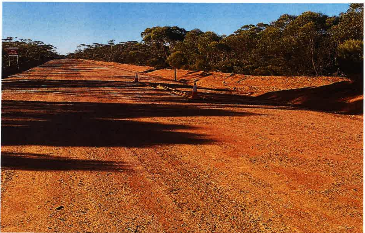
Rut in road approaching railway line from the south
