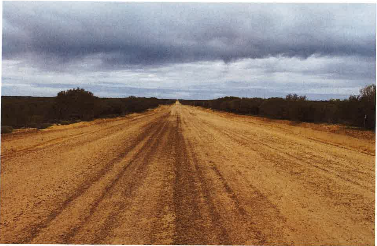
View of road passing through a gravelly sand area showing some minor corrugation development
