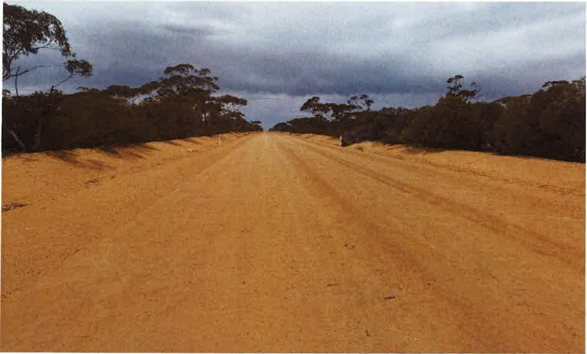
View of road at 91km mark showing excellent condition of both cross-sectional shape and surface
