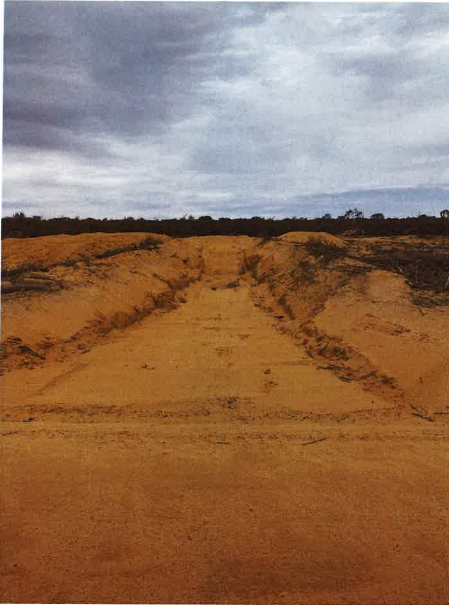
Deep perpendicular drain designed to move water away from road and ensure seepage under road surface is minimised
