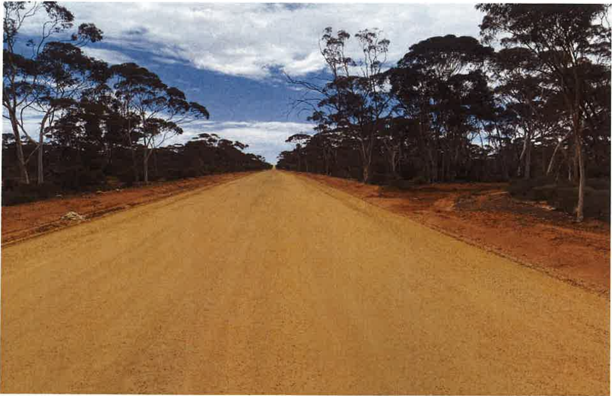
View of gravel sheeted section through previously clay surfaced area, road has good shape too
