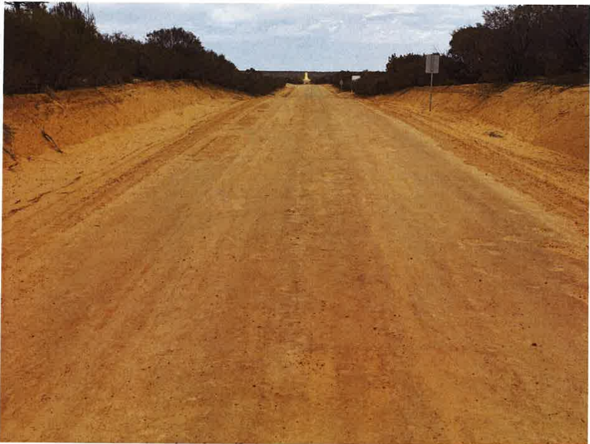
View of sandy section of road looking south at the 94km mark, showing shallow potholes
