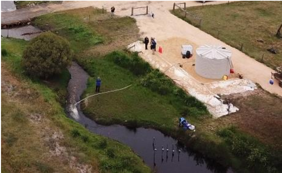
Figure 4: Clay storage tank and dosing pumps at the treatment site on Punrak Drain.
