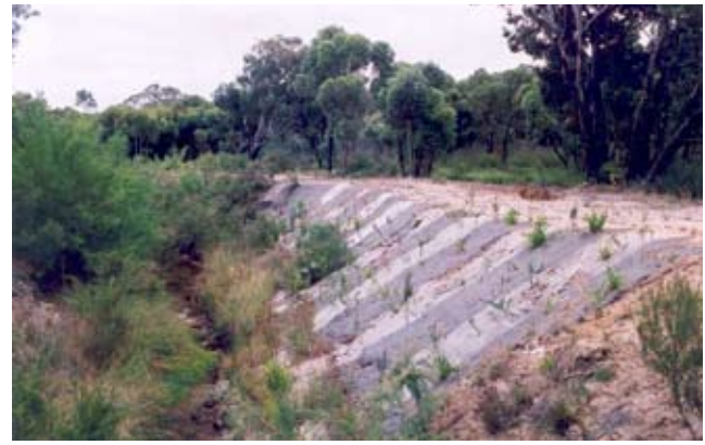
Figure 21 Revegetation work being undertaken on Cuppup Creek. The matting helps stabilise the banks whilst the plants grow.
