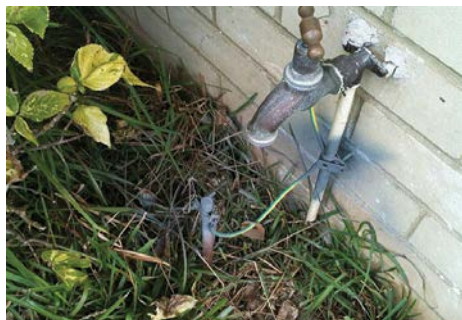
Green and yellow earth wire attached to metal stake
