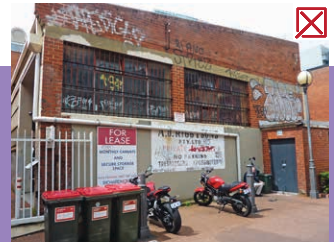
Photo 2.35 Placement of bins near gate and horizontal downpipe may provide easy access to vandals.
