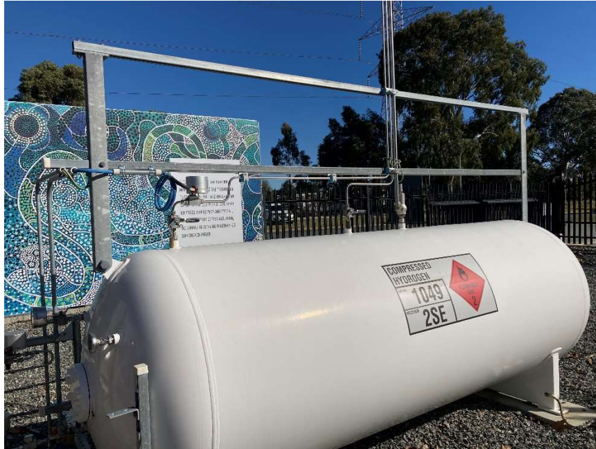
Figure 2. Hydrogen Storage Tank
