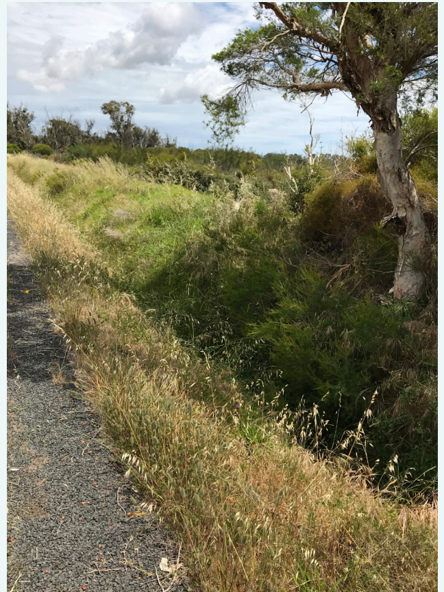
A roadside drain. These drains help to quickly transport water from the road to larger drains, November 2020.
