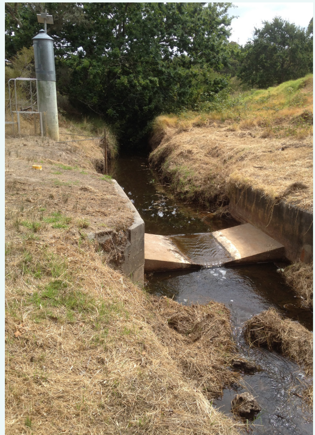
The weir and gauging station at the Mill Brook sampling site. The exotic grass along the brook has been cut back, January 2017.
