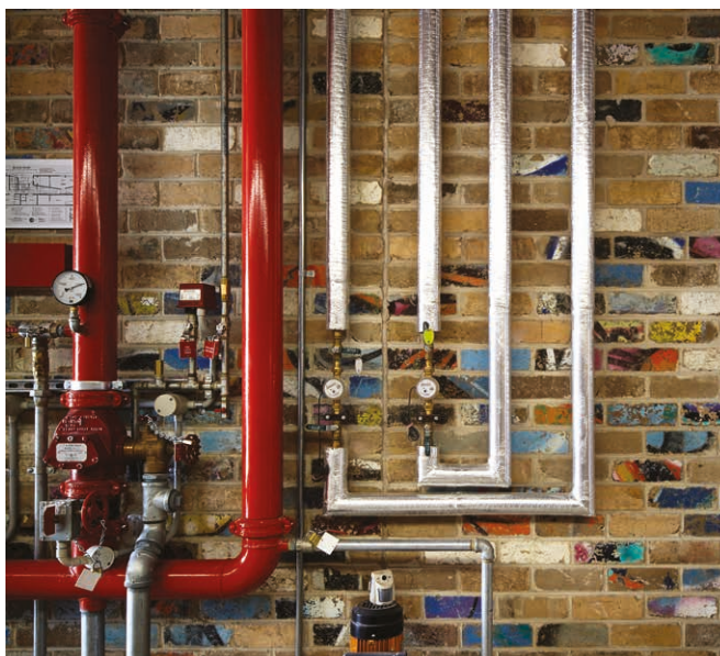
Photo 4.18a This apartment building has incorporated service facilities into the design by making it visible and prominent and a feature along the internal wall. (PC)
