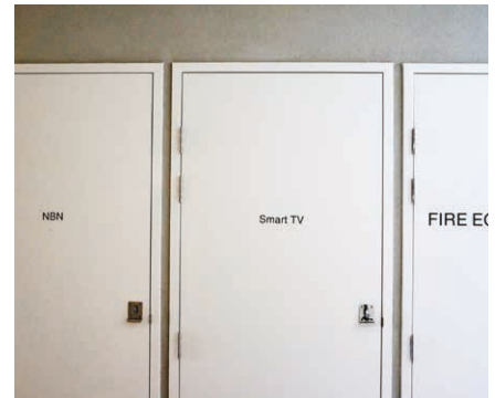
Photo 4.18b This apartment is fibre-to-premises ready.
