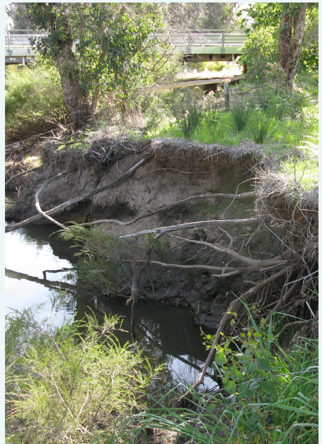
Bank erosion near the Upper Preston River sampling site. Erosion like this can add particulate matter to the river during high flows, October 2009.
