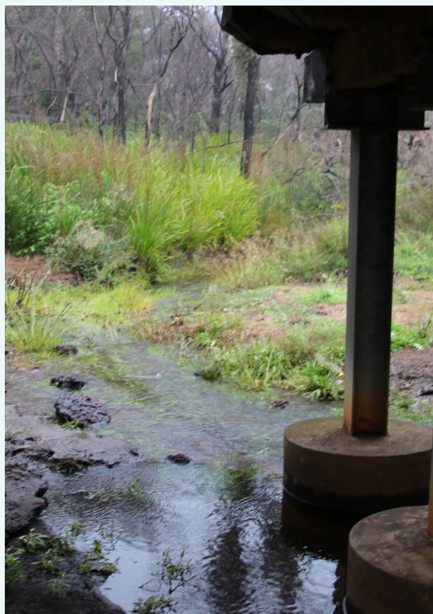
Looking downstream along West Bay Creek from underneath the West Bay Creek Road bridge, June 2019.
