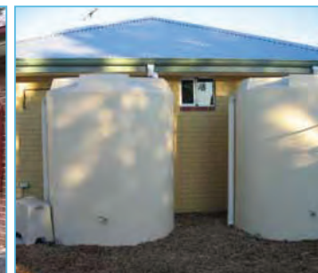
Poly domestic rainwater tanks
