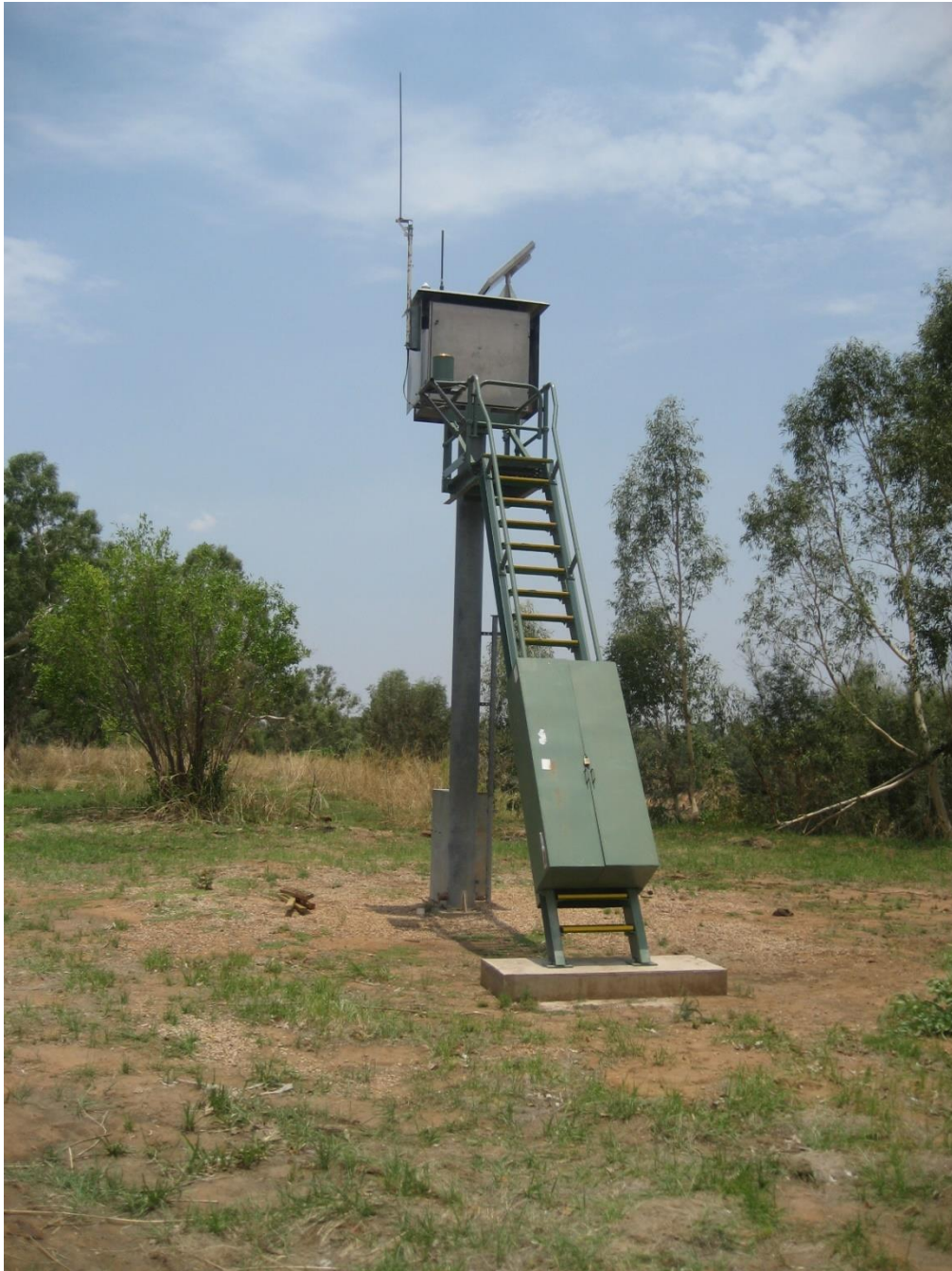
Figure 21 Gauging station infrastructure at Noonkanbah on the Fitzroy River
