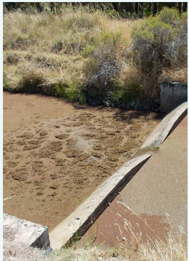
High nutrient concentrations encourage macrophyte growth. Here the drain is completely covered by macrophytes, December 2014.
