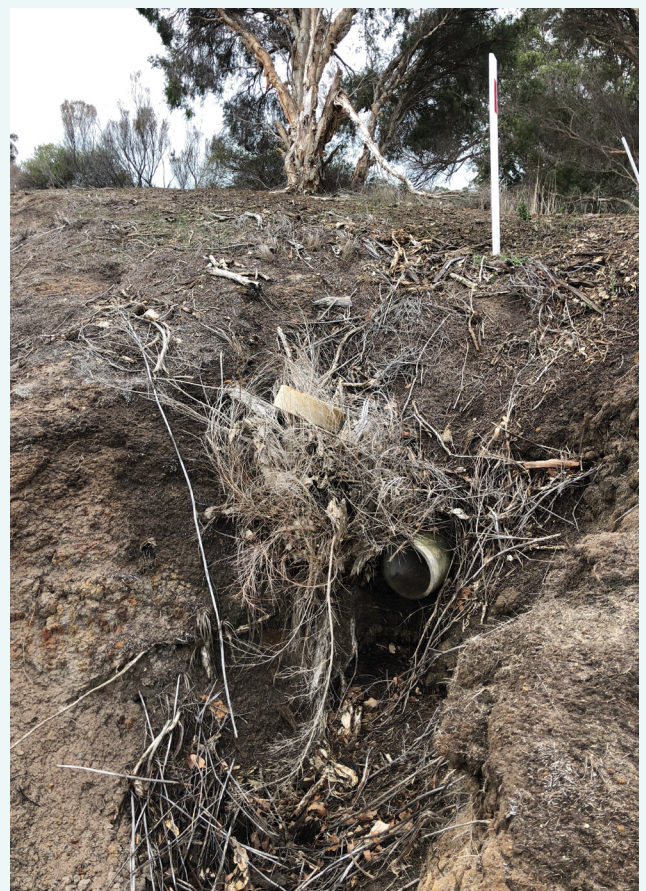
Pipe discharging into Cuppup Creek, June 2018.
