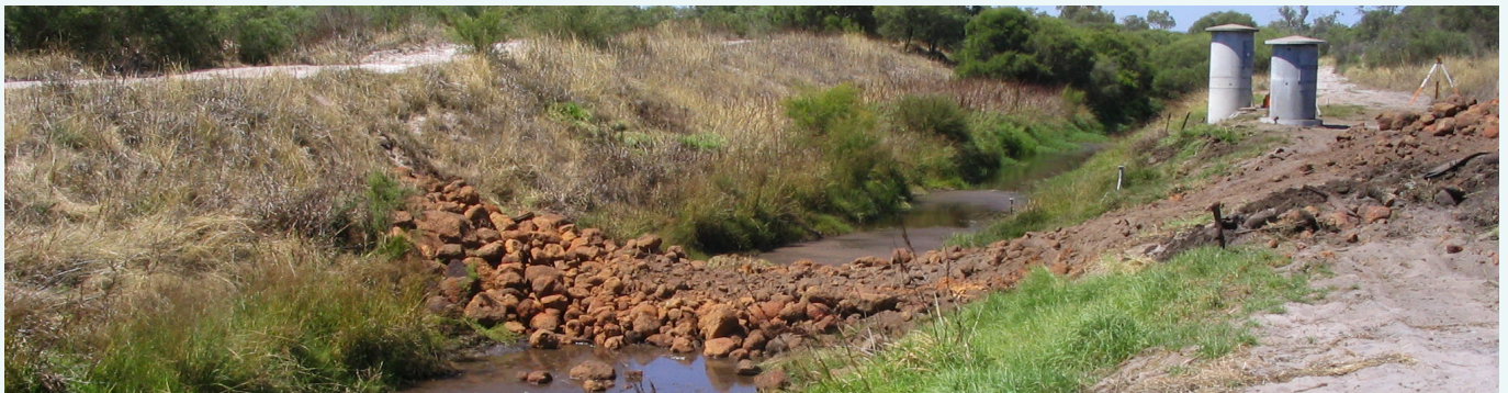
The rock weir used for gauging at the Punrak Drain sampling site under construction, March 2006.
