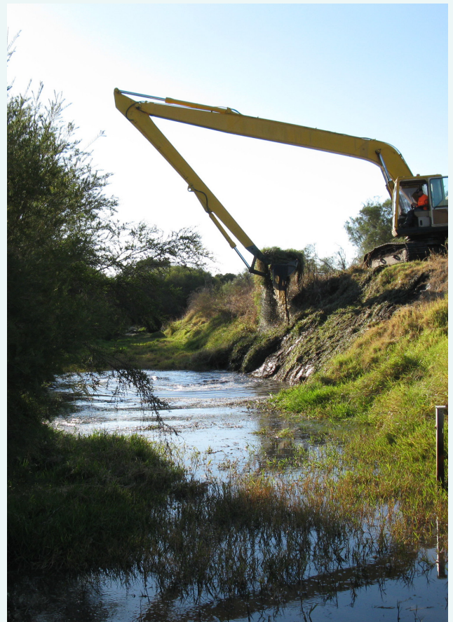
An excavator removing excess plant growth from the drain close to the sampling site, May 2020.
