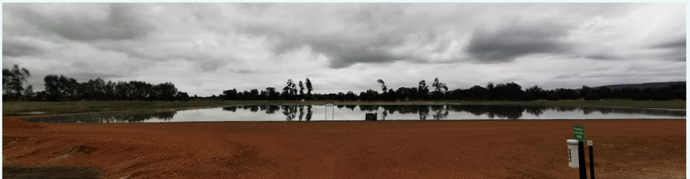
A treatment pond at the Waroona Waste Water Treatment Plant, September 2020.
