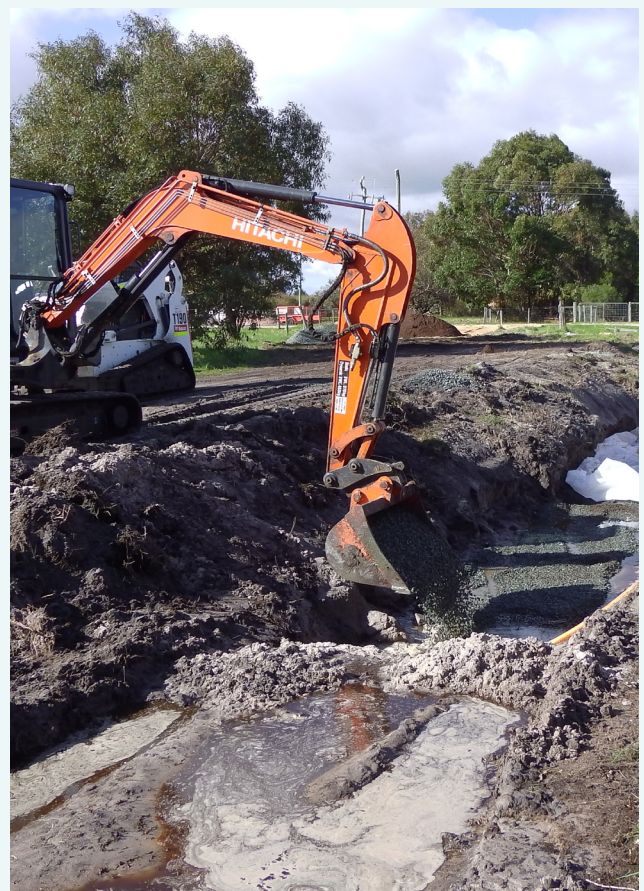
Installing treatment beds in Gull Road Drain that use a high phosphorus-adsorbing material to remove some of the phosphorus from the water, August 2017.
