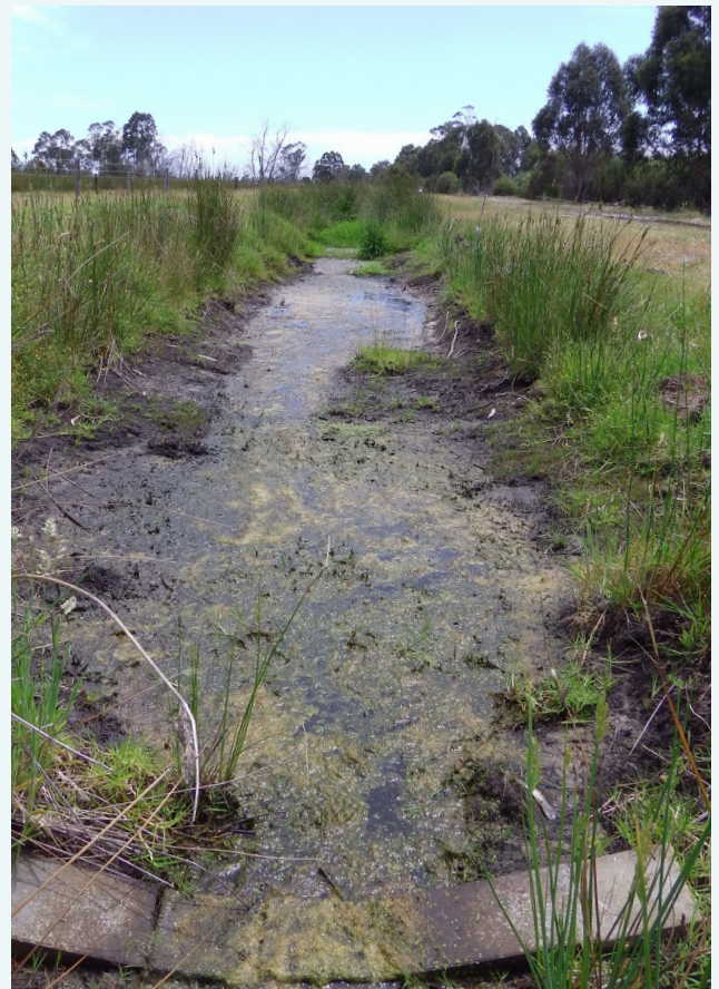
Algal growth in the upper part of Gull Road Drain. High nutrient concentrations contribute to excess algal growth such as this, November 2017.
