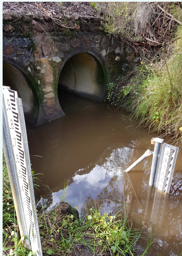
The culverts under the bridge at the Little River sampling site, June 2017.
