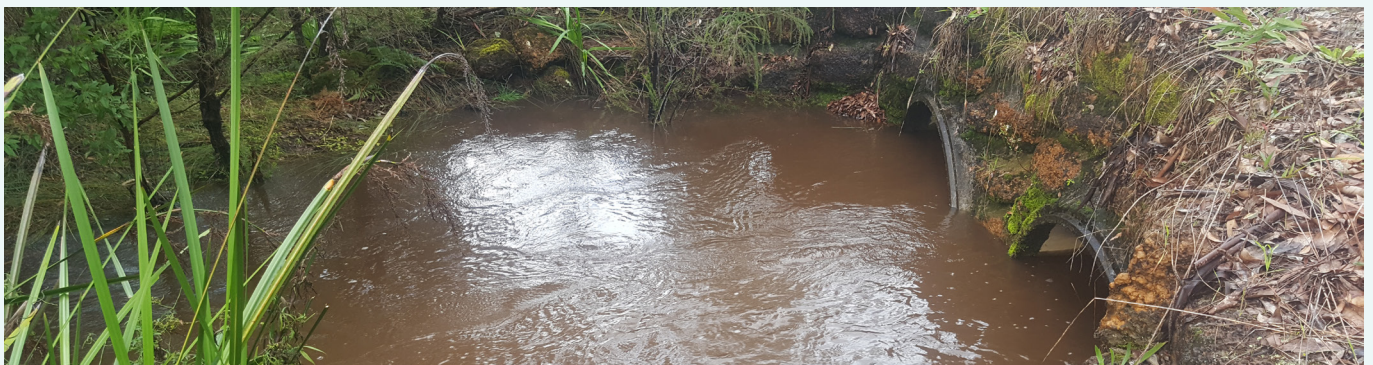
The culverts at the Little River sampling site during high flow, August 2018.
