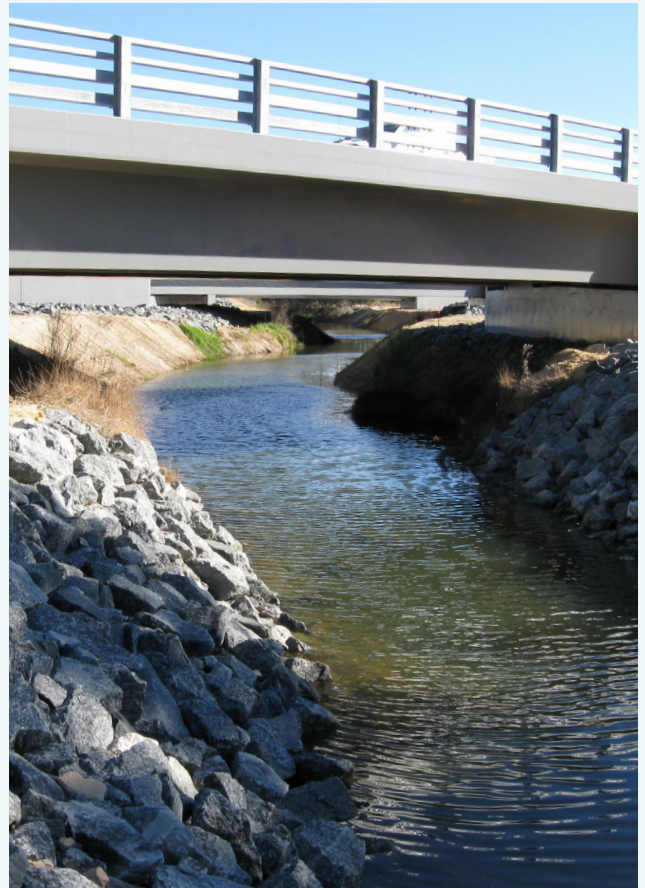
Stabilisation works undertaken on Mayfield Drain to help prevent bank erosion. This photograph was taken at the same location as the one of the previous page, June 2009.
