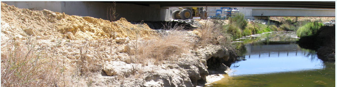
Mayfield Drain at the Forrest Highway bridge. Note the erosion and undercutting of the bank on the left side of this photograph, March 2009.
