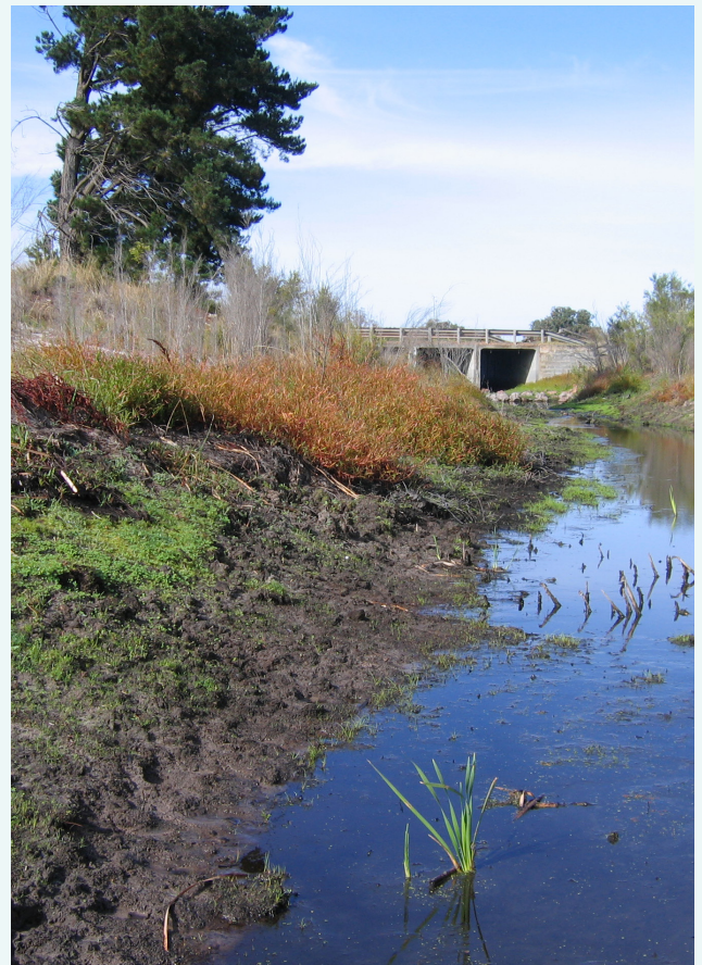
Excess macrophyte growth has been removed from the left bank in the foreground of this picture, leaving an unprotected bank which is prone to erosion in high flows, May 2020.
