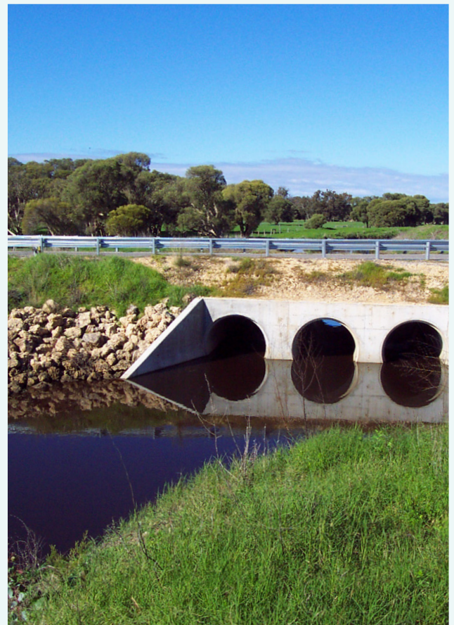
The culverts where Peel Main Drain passes under Karnup Road near the sampling site, July 2002.
