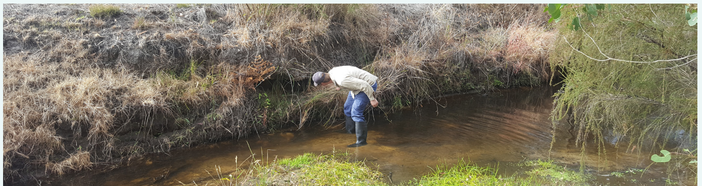
Examining bank undercutting along the Sleeman River, April 2018. This undercutting is caused by erosion which occurs because of a lack of fringing vegetation which helps stabilise banks.
