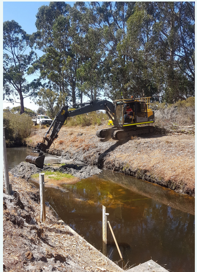
Removing the sand deposit in the weir pool at the Sleeman River sampling site, February 2019. This was done to improve the gauging station's ability to measure flow.
