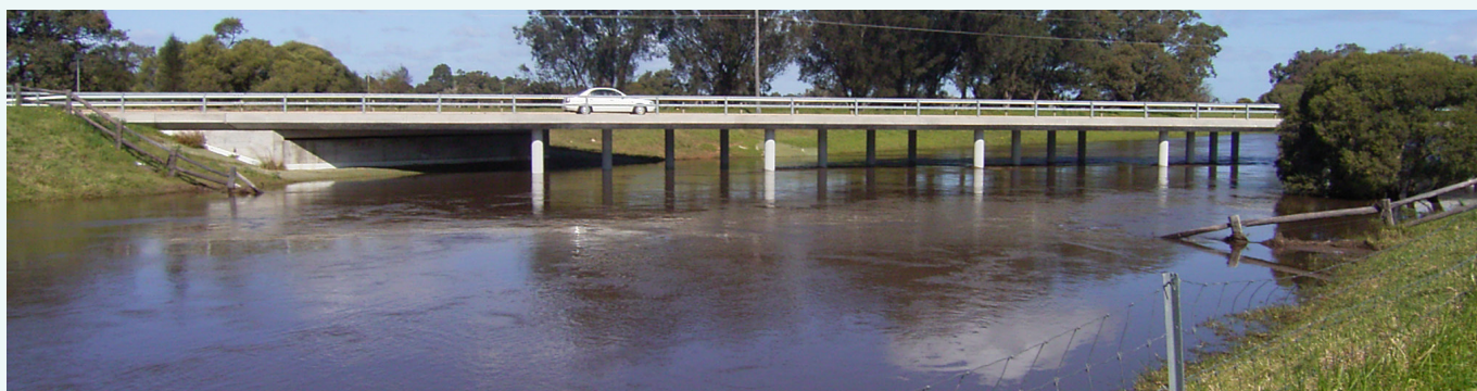
The Serpentine River flowing under Karnup Road Bridge during high flows, August 2005.
