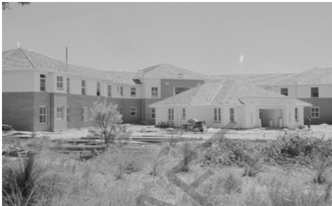
Archival Image 2: The new Infectious Diseases Hospital administration and ward buildings nearing completion in 1938 (Source: SLWA online image call no.095479PD)
