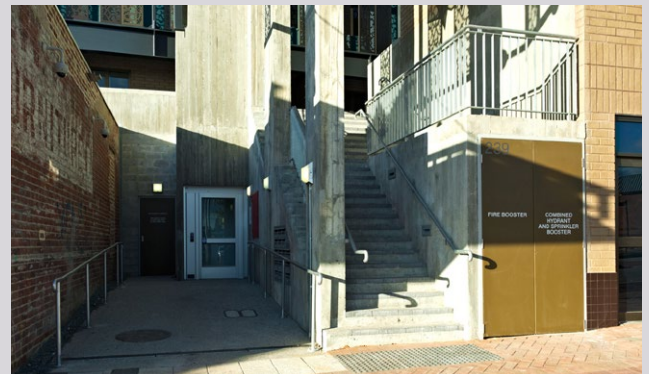
An example of the fire hydrant booster discreetly integrated within the building envelope
