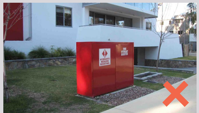
An example of the fire hydrant booster with a poorly designed outcome
