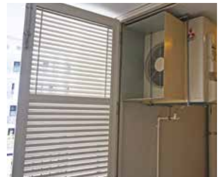
Photo 4.18c Carefully located and well-ventilated covered recess to conceal air-conditioning condenser unit.
