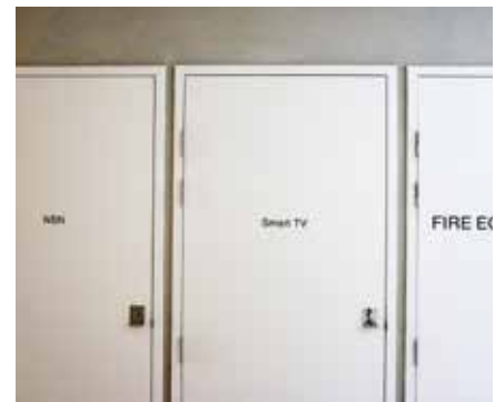
Photo 4.18b This apartment is fibre-to-premises ready.
