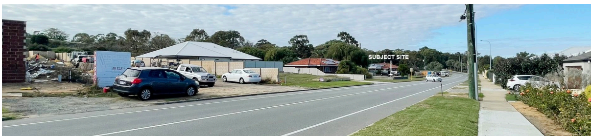
Photograph 8: Standing on western side of Rockingham Road, looking south east towards construction works underway of R40 development site.
