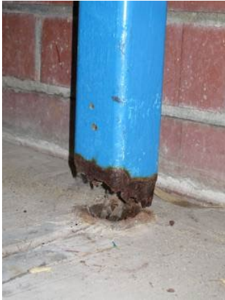
Figure 7: Potential effects of poor corrosion protection.
