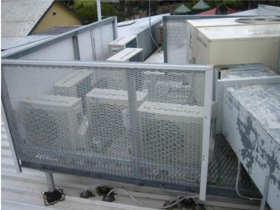
Figure 8: Example of poorly accessible mechanical equipment
