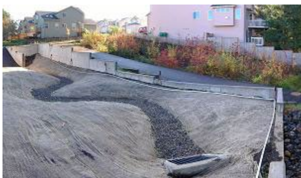
Figure 1: Two bio-swales for a housing development. The one in the foreground is under construction, while the one in the background is already established. Image source: Wikimedia
