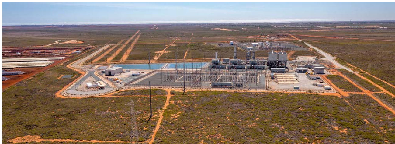
South Hedland Power Station, within Boodarie strategic industrial area. Imagery courtesy of DevelopmentWA.
