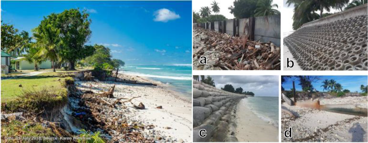
Figure 15: Recent erosion at West Island settlement (circa 2021) and coastal protection structures introduced to protect the West Island settlement (a) older vertical seawall (b) Seabee seawall (c) GSC revetment and (d) older groynes (RHDHV, 2021a)
