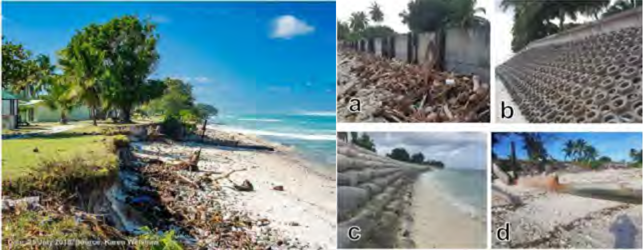
Figure 15: Recent erosion at West Island settlement (circa 2021) and coastal protection structures introduced to protect the West Island settlement (a) older vertical seawall (b) Seabee seawall (c) GSC revetment and (d) older groynes (RHDHV, 2021a)
