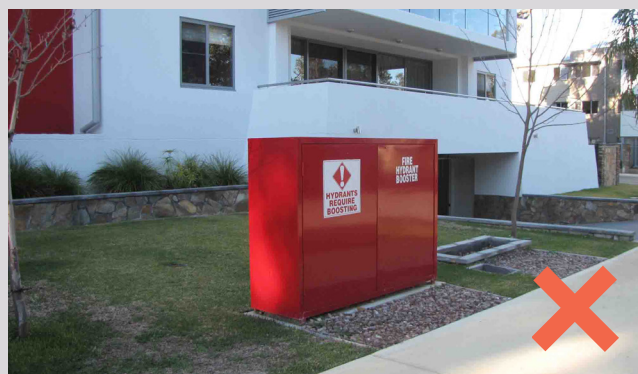
An example of the fire hydrant booster with a poorly designed outcome
