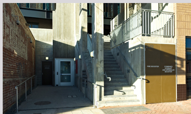
An example of the fire hydrant booster discreetly integrated within the building envelope
