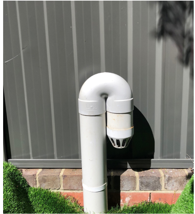
Photo 2: Example of low level vent termination
