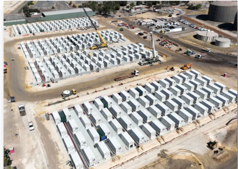
Synergy 200 MW / 800 MWh Kwinana BESS 2, connected in 2024 as Grid Following under present SWIS regime.
