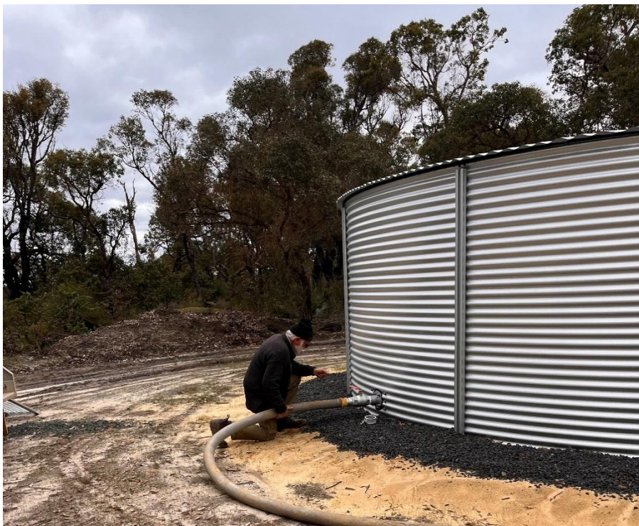
Tonebridge fire emergency tank
