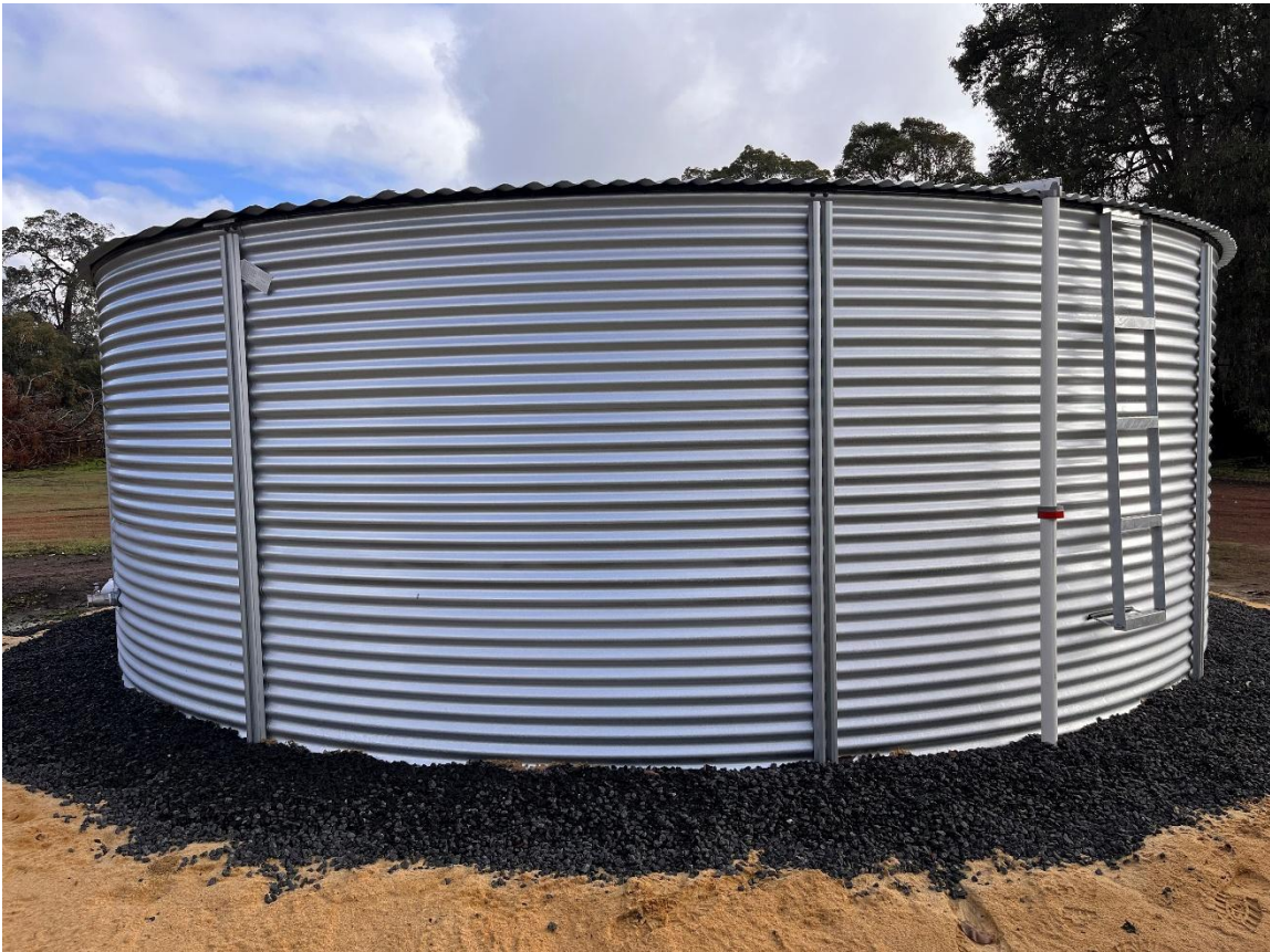
Wilga Hall fire emergency tank
