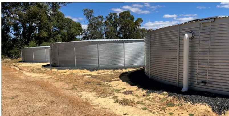
Three of the six tanks at the site
