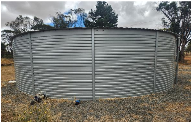
Broomehill town dam tank
