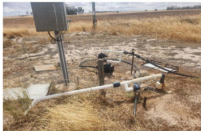
Bore and outlet
