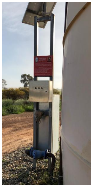
Swipe card standpipe system
