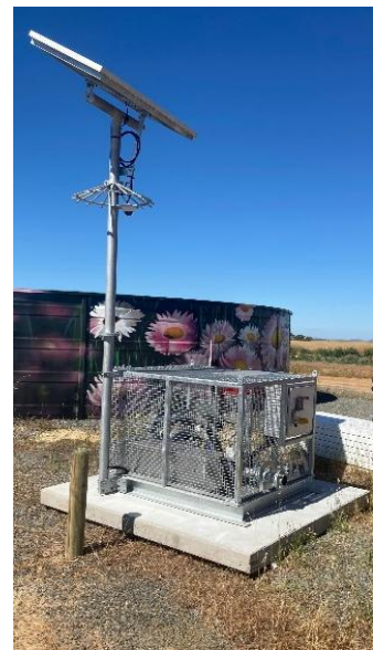
Tank, electric swipe card and pump for bore
