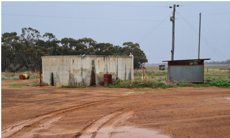
Anderson's Bore 1 tank and pump/bore housing (June 2022)
