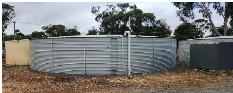
Tambellup Shire Depot tanks 3 and 4
