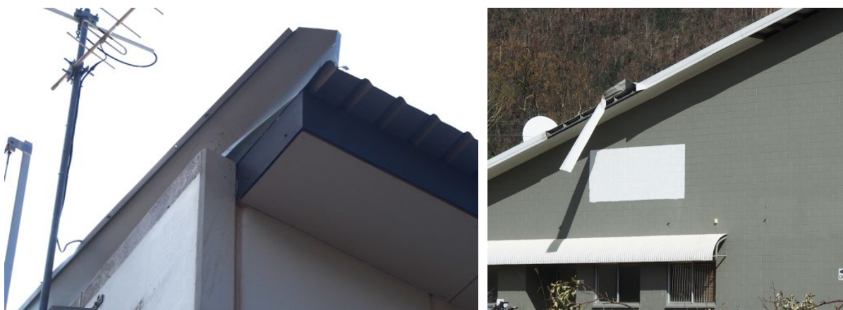
Figure 8.1 Lifted flashings after high wind events
