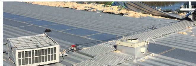
Air conditioner led to damage
