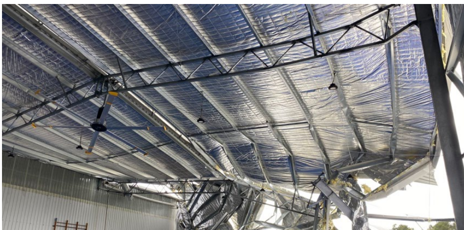
Figure 8.6 Failure of lightweight trusses triggered by buckling of bottom chord
