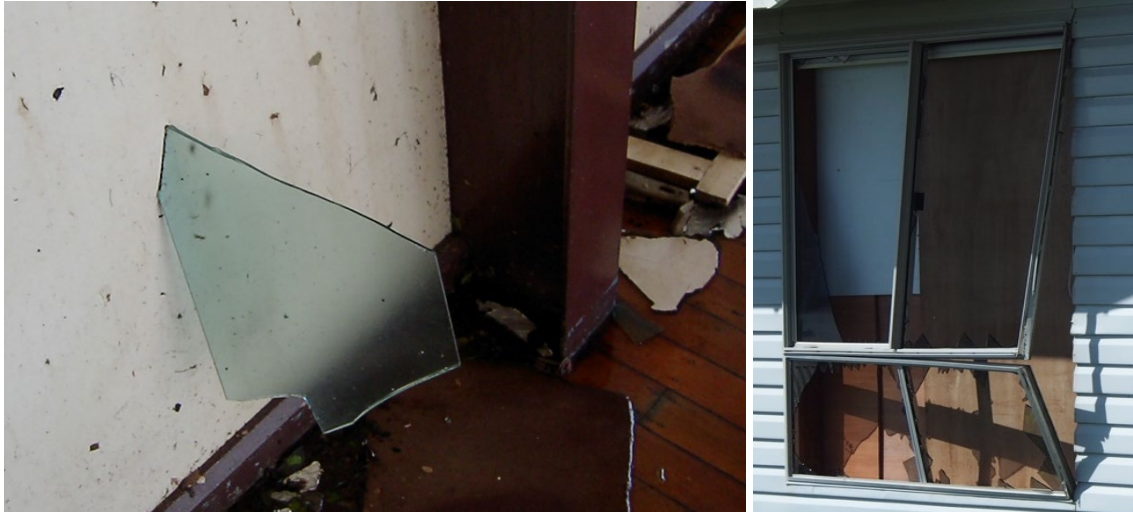
Figure 8.9 Float glass embedded in a wall after glass failure & window sucked out of building
