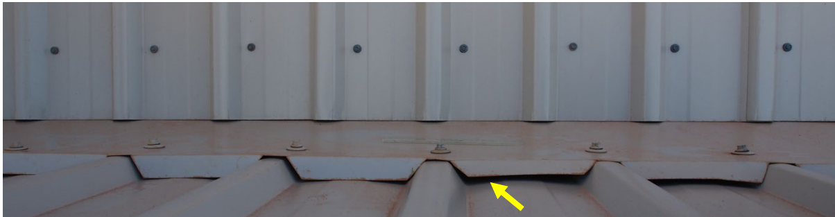
Figure 8.2 Water penetration under well fastened flashings
