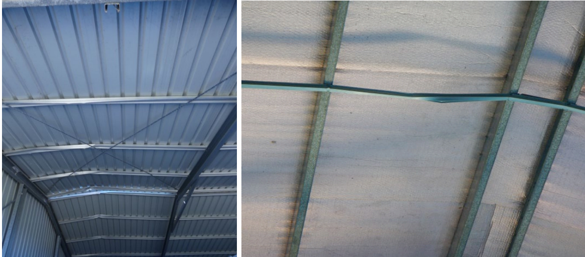
Figure 8.5 Purlins with lateral-torsional buckling and buckling of the bridging
