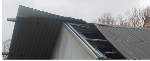
Satellite aerial led to damage
