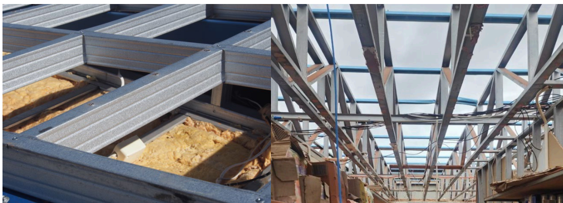
Figure 8.4 Failures because of low thickness of steel in purlins or battens
