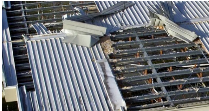
Figure 8.3 Failure of part of secret-fixed roofing due to problems with clips
