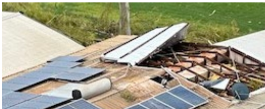
Solar panels led to damage
