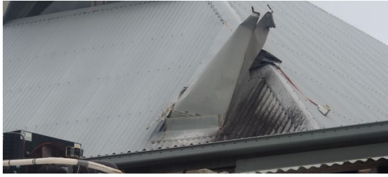
Extractor fan led to damage
