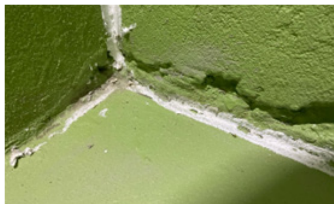
Figure 1: Poorly prepared wall/floor junction in shower and incorrectly applied bond breaker fillet.
