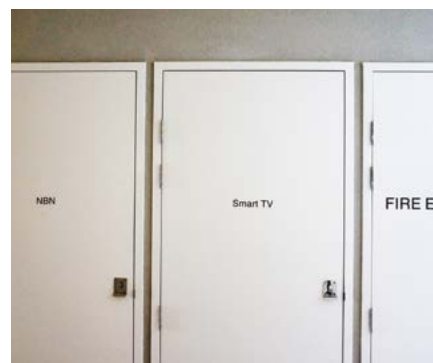
Photo 4.18b This apartment is fibre-to-premises ready.
